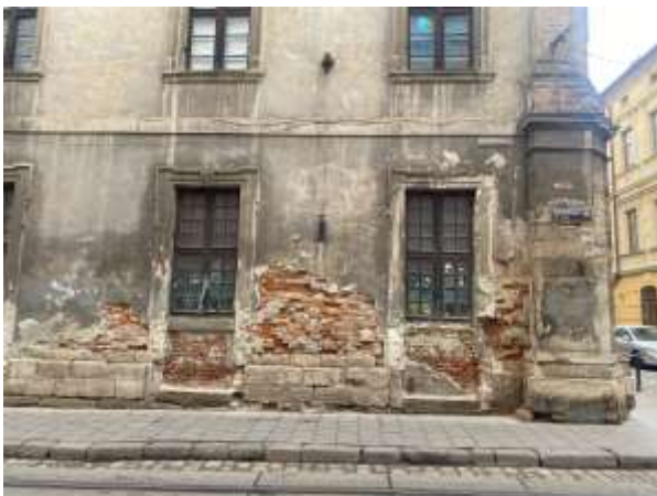
Fig. 1. Damaged masonry walls of historical heritage buildings situated on Rynok Square in Lviv. Photo by M. Melnyk
