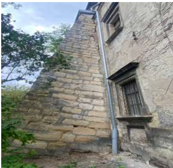
Fig. 2. Bernardine Church in Lviv counterforces and walls structural damages. Photo by M. Melnyk
