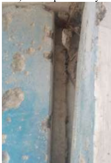
Fig. 3 Damaged wall panel No. 1, displacement of 26 cm (view from the balcony side).
