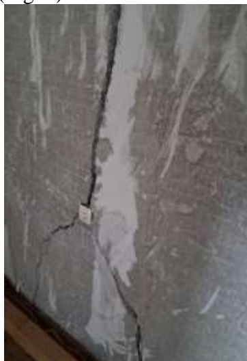
Fig. 4 Damaged wall panel No. 3.
