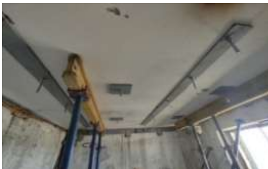
Fig. 11 Scheme for strengthening the floor slab between the 10th floor and the technical floor.
