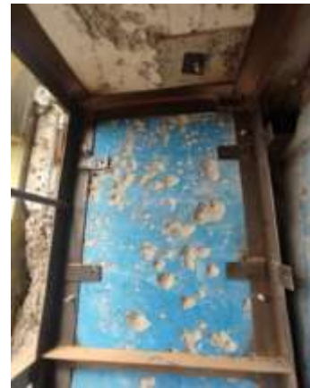
Fig. 12 Steel frame for the restoration of the balcony structures. Photo by Dmytro Levkivskyi
