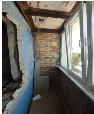
Fig. 13 Steel frame for the restoration of the balcony structures. Photo by Dmytro Levkivskyi
