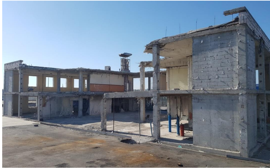
Fig. 2. General view of the partially collapsed building
