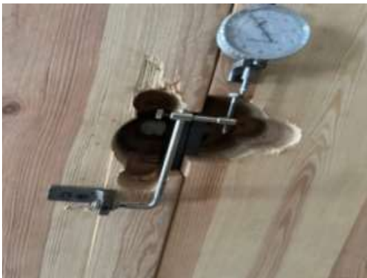
Fig. 15 Failure of bolt M20 and enlarged hole milled in the timber for bolts M24. Photo by Andrii Bidakov
